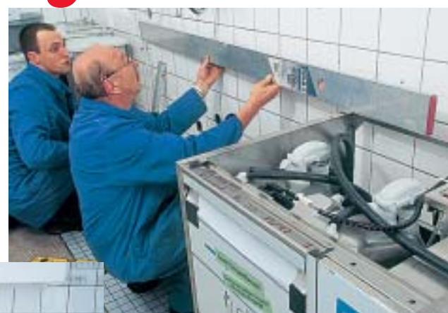
Installation and connection of the Meiko TopLine 40 E to the building's supply and waste disposal systems
